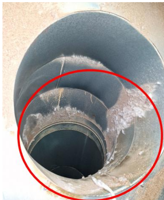
Figure 10: Excessive Trash & Dust Deposition in Humidification Plant Filter Room
